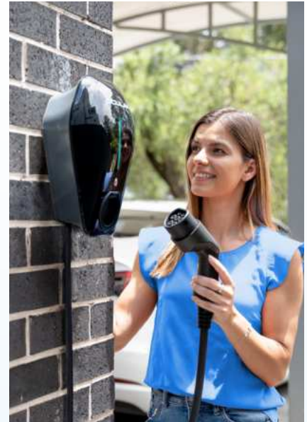
IQ Home Solar Installation
